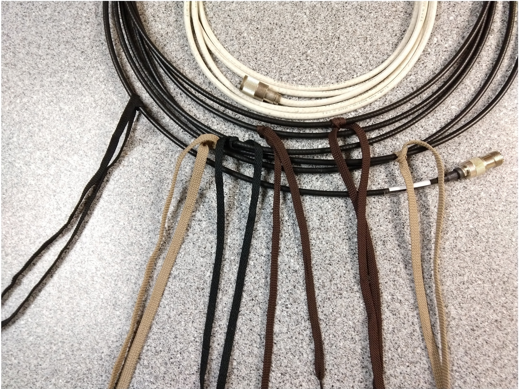
coax cable with mast ties
